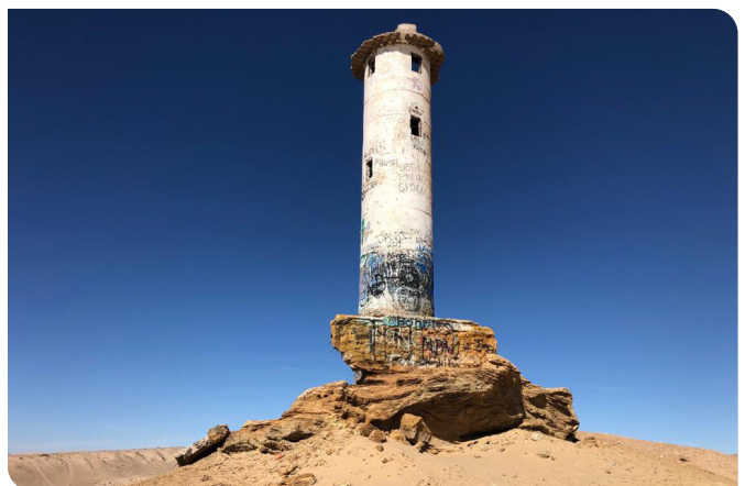
A temporary light source was installed off-site when the old Machorro Lighthouse was deemed a safety risk.
