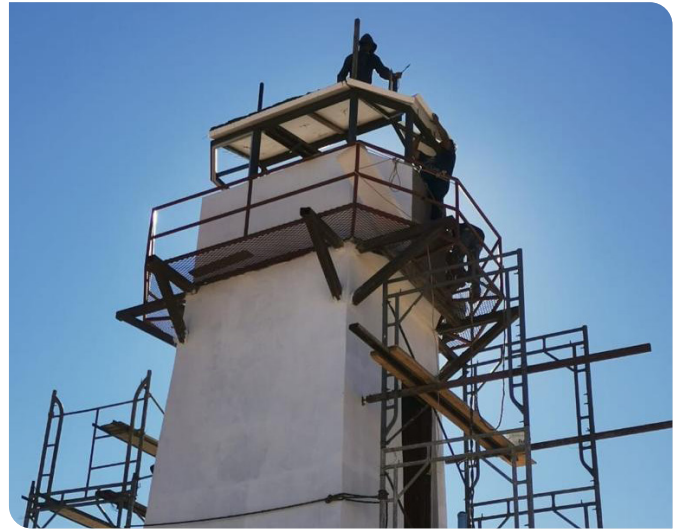
Construction of the new Machorro Lighthouse was complete in only 45 days and included Sealite's SL-300 Solar LED Long Range Marine Lantern.
